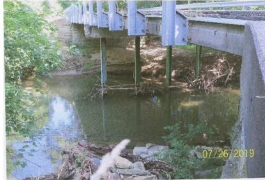
Channel Photo is not acceptable, due to sharp angle. Cannot see channel relative to abutment on the right, or the channel immediately upstream of the bridge.
