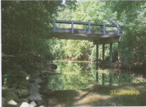
Channel photo could have better visibility of abutments. Fortunately the channel is narrow enough here to see the abutments are set well back from the channel.
