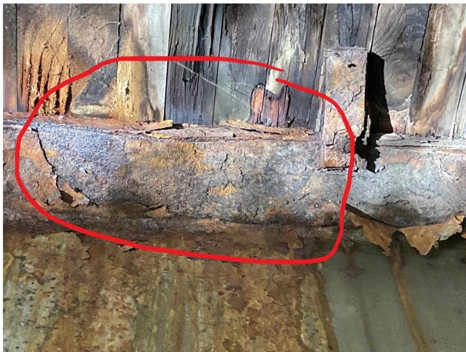
The upper flange is not much better and is hard to see in the darkened areas.
